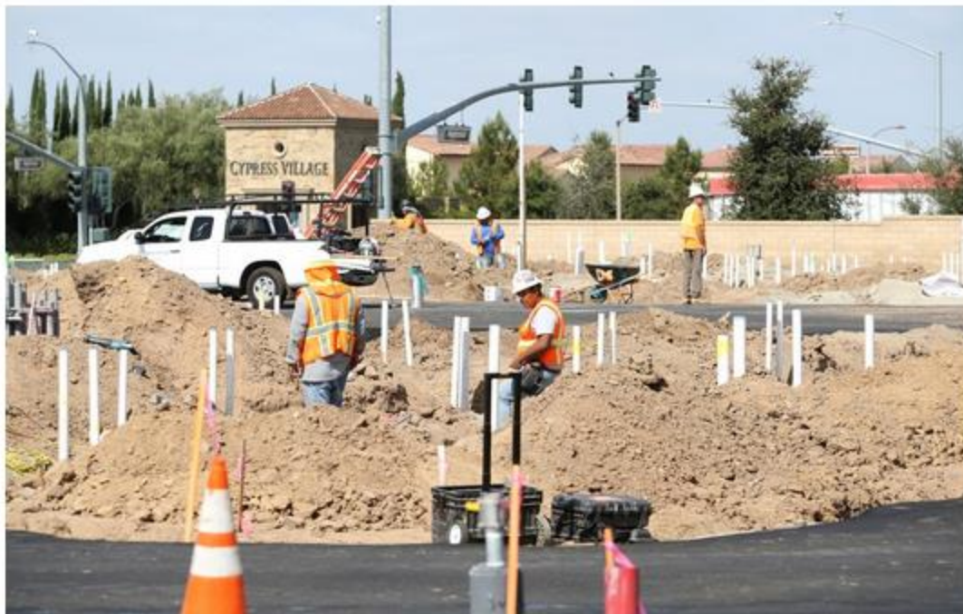
Construction is now underway for an affordable housing development near the Orange County Great Park in Irvine. (Don Leach / Staff Photographer)
